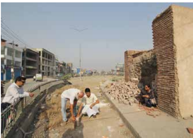
Fig. 2: Citizens Site Visit 14 May 2017. Showing raft distance at 3.4m of Hydraulic Works. Blatant Violation of 200 foot Buffer Zone. Photo: Maria Waseem
