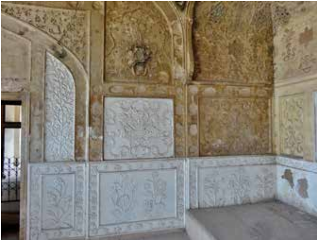
Fig. 5: Poor quality of restoration in a room of the Lahore Fort. Photo: Zulfiqar Ali Kalhoro
