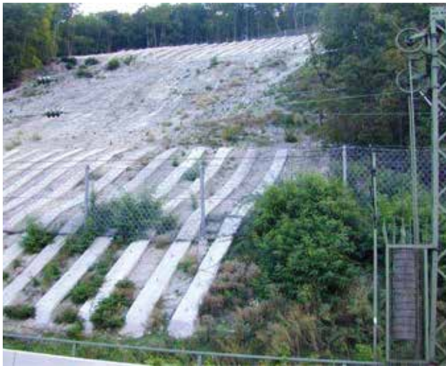
Fig. 3: A slope near Boppard has been concreted in order to prevent further landslides. Photo: Bürgerinitiative Rheinpassagen
