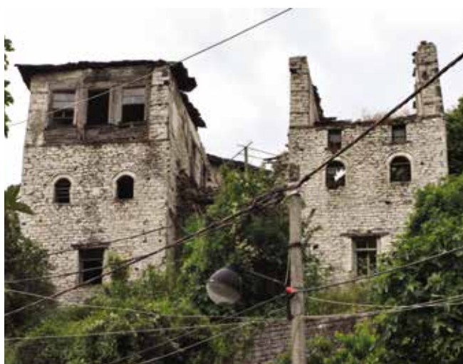
Fig. 4: A large number of vernacular houses protected as cultural monuments are rapidly deteriorating and in need of emergency intervention. Photo: Stephan Doempke
