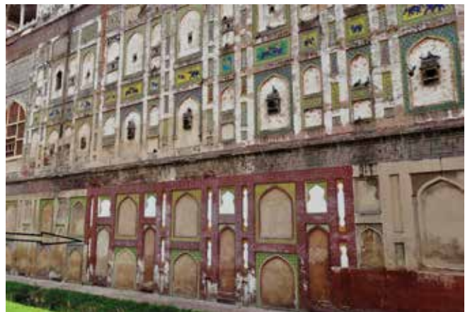
Fig. 2: Panels of the lower part of the wall have been cemented. Photo: Zulfiqar Ali Kalhoro
