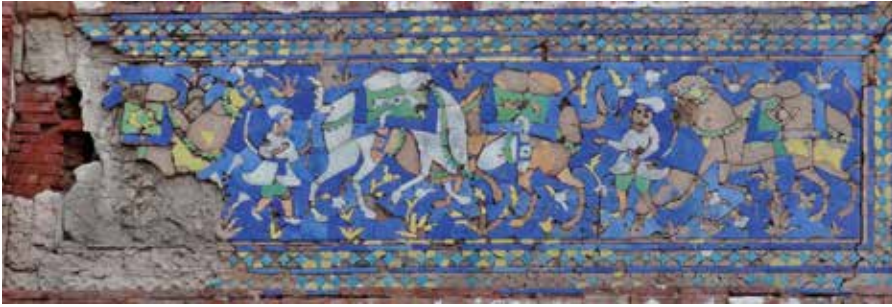
Fig. 4: A tile mosaic in bad state of preservation.
