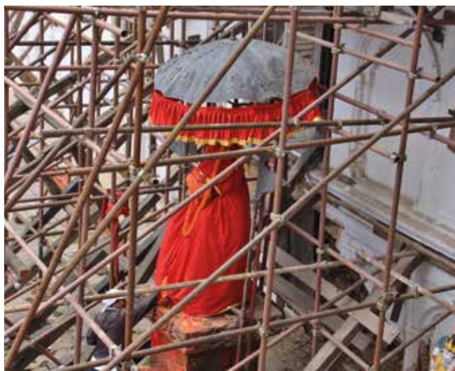
Fig. 2: 17th century Hanuman statue within the temporary shoring at Hanumandhoka. Photo: Alina Tamrakar
