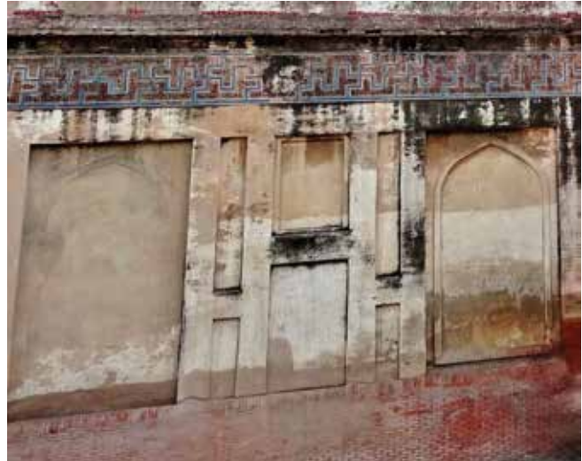
Fig. 2: Panels of the lower part of the wall have been cemented. Photo: Zulfiqar Ali Kalhoro
