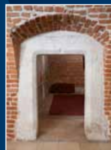
Renaissance portal and window architrave in the Villa Decius cellar and basement
